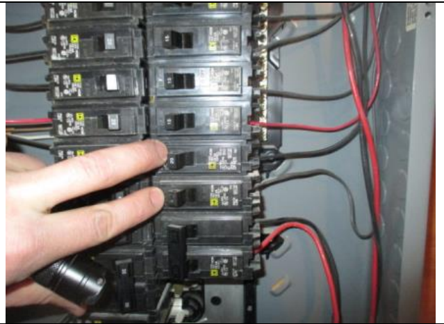
14 gauge wire on 20 amp breaker circuit, recommend further evaluation by licensed professional.
