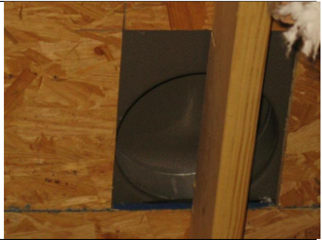
Roof louver visible from inside the attic. A wire screen may also be placed over this opening if pest intrusion is an issue.
