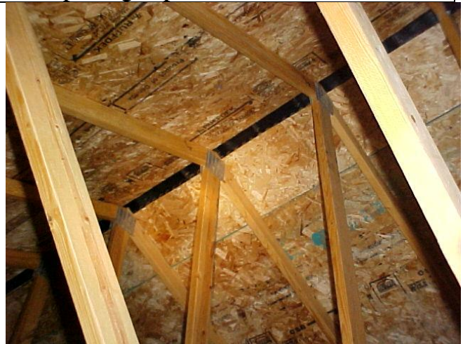
Notice the separation of decking at the center of the peak, this allows air to escape the attic space through the ridge vent.
